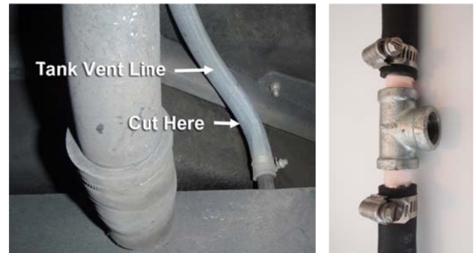
Tank Vent Line
